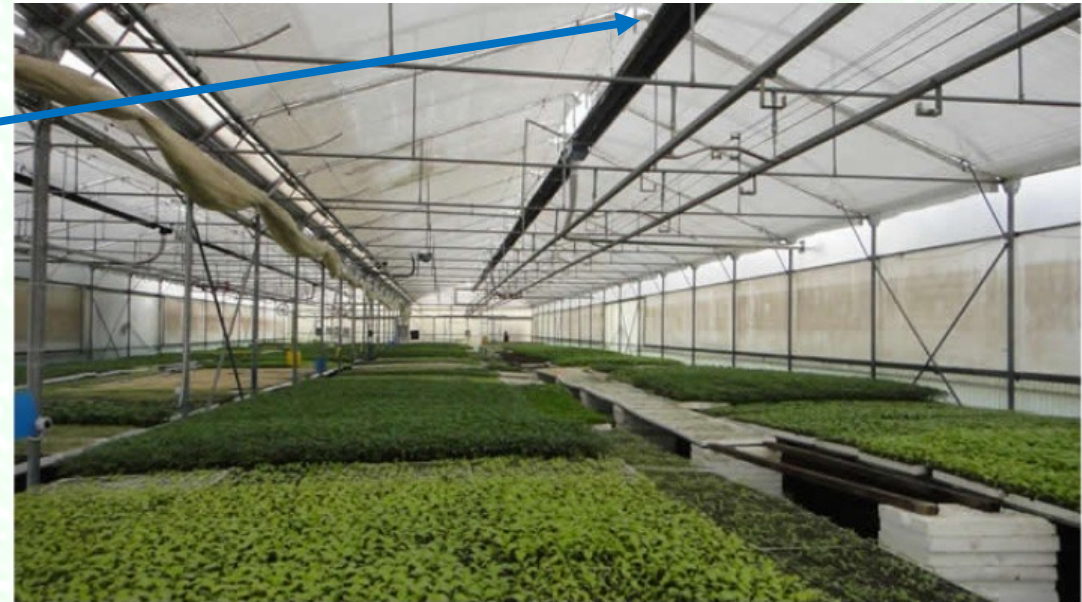
System of gas-fired IR radiators comprising of six radiant tubes, of 18 m length and of 45KW thermal power each, placed at a height of 3.0 m above the plant canopy in an arched greenhouse in the region of Koropi, Attica, Greece.
