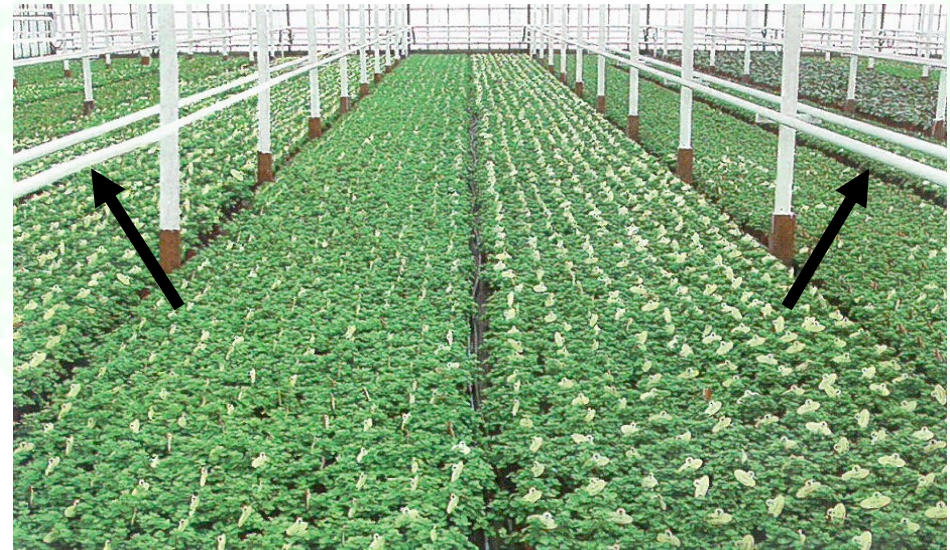
Heating pipes on the periphery and inside the greenhouse
