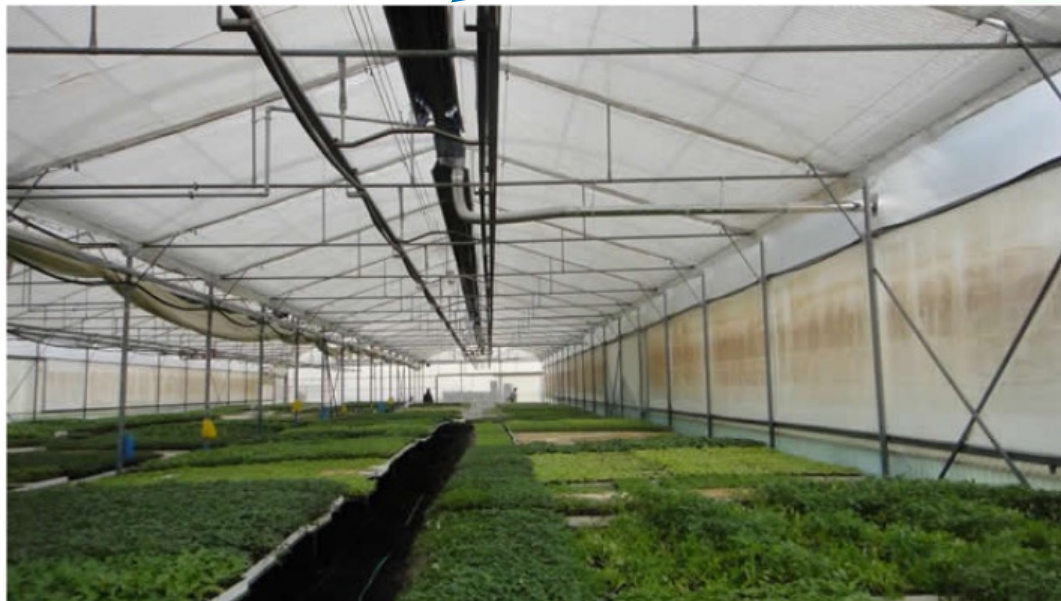
Infrared heating systems type INFRA MONOTUBO 18MI, heat capacity 45KW each, powered by LPG (Propane) fuel ( www.natural-gas.gr )
