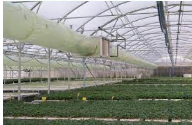
Plastic perforated pipes hung from the ceiling
